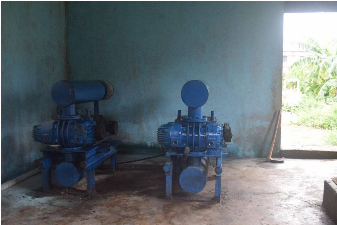
Liquid waste management plant
